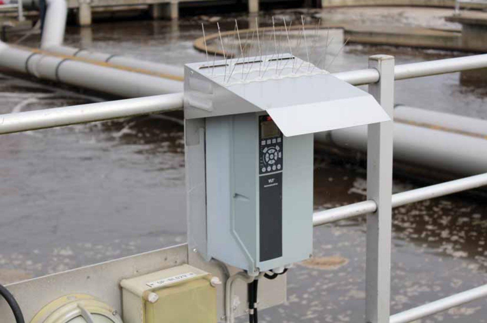
Activated sludge nitrification & denitrification: 16 VLT® drives rated 4 kW with PROFIBUS, RFI filter, IP66 enclosure rating and climate shield control the aeration mixers.
