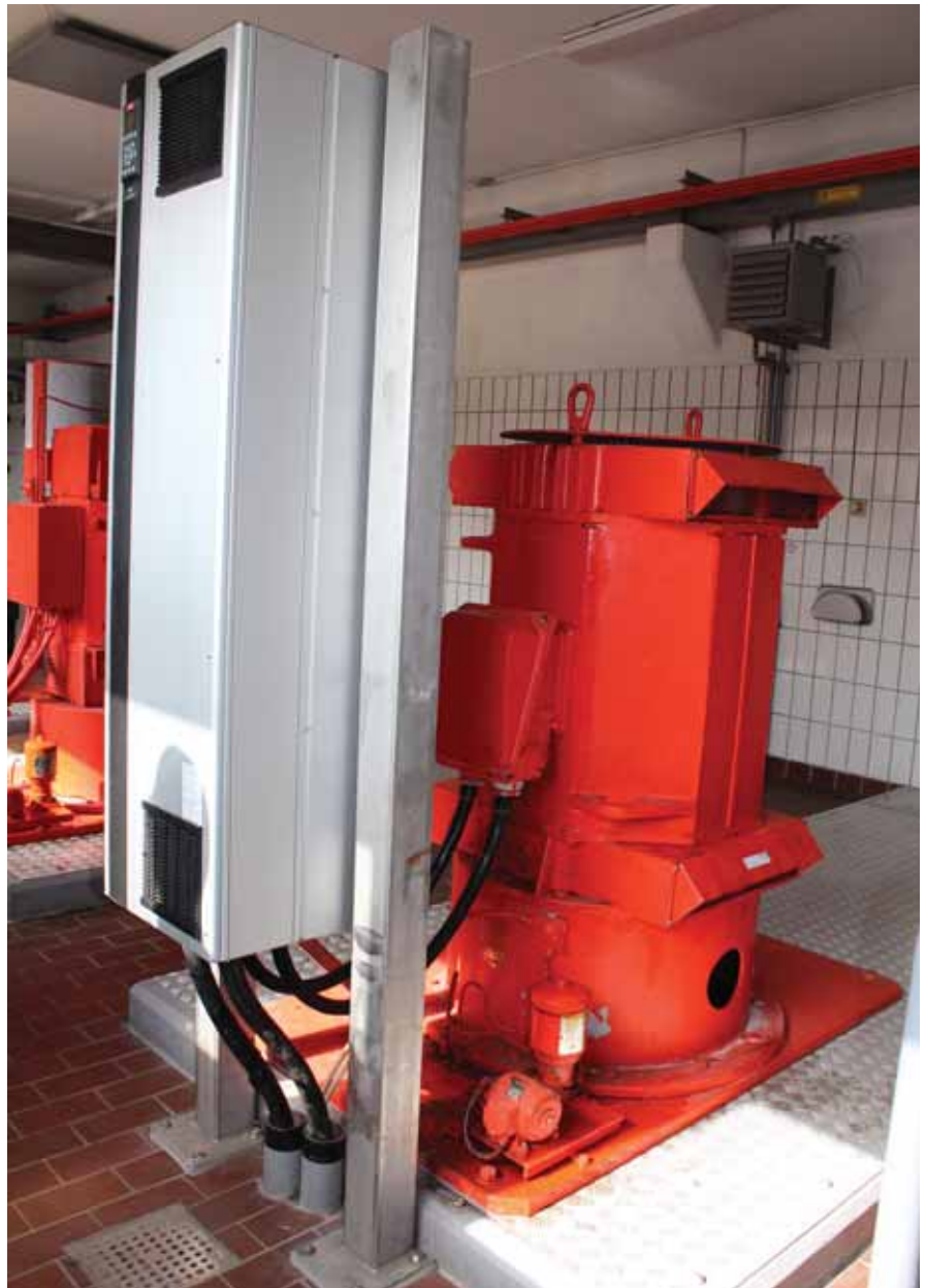
Discharge pumping station: A VLT® rated 160 kW with IP54 enclosure controls this pump weighing 1.25 tonnes
