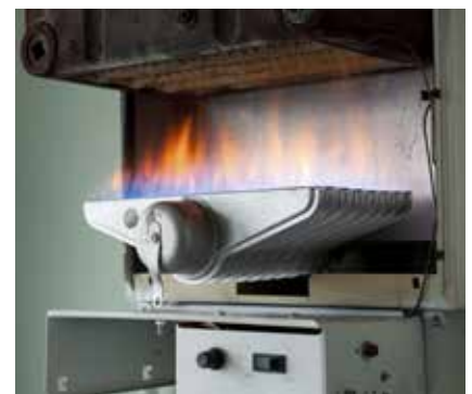
Individual air-conditioning units (top) and gas boilers (bottom) are just two of the technologies that district energy can replace.
